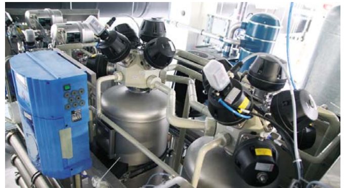
Ion exchanger with GEMÜ multi-port valve block
